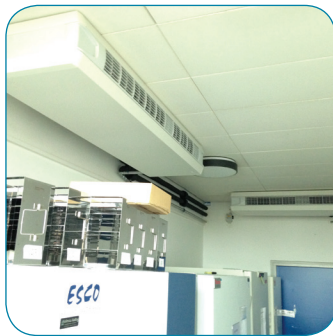
To fan coils
